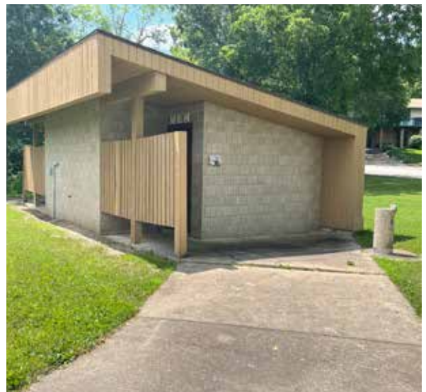
Restroom facilities (Update)
