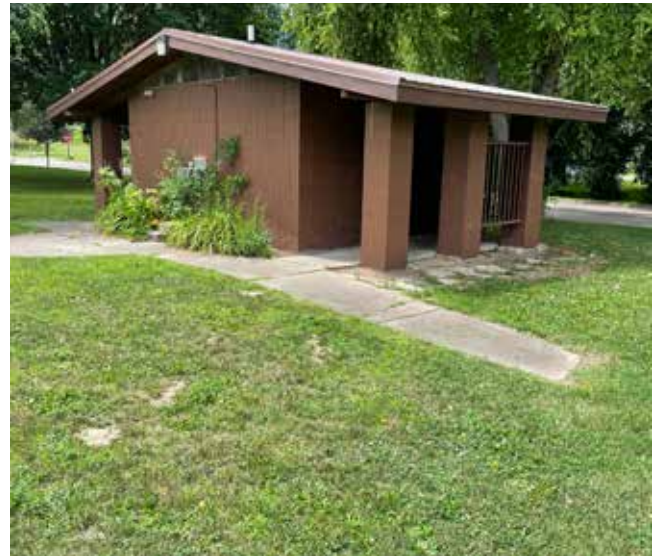
Existing non-ADA compliant restroom building with no sidewalk access
