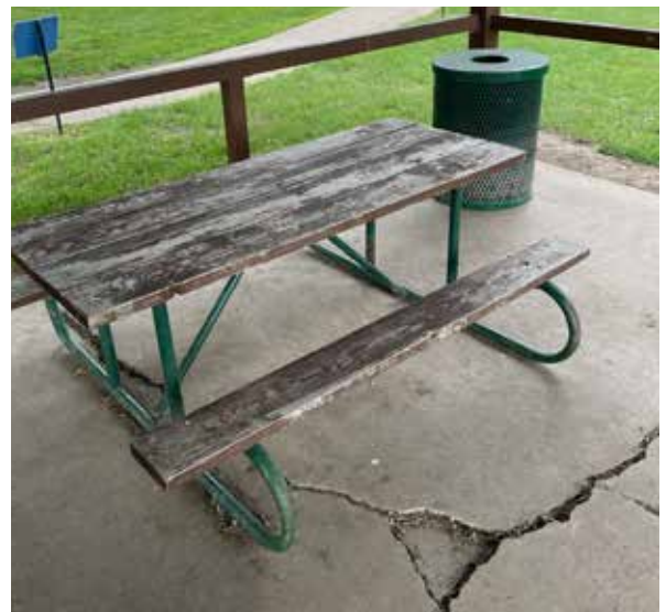
Cracked concrete in small picnic shelter (Repair)
