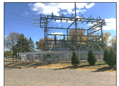
Xcel Energy Electrical Substation near Beach Park
