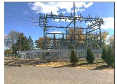
Xcel Energy Electrical Substation near Beach Park
