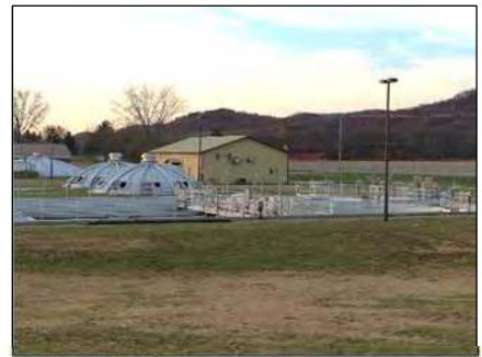
Wabasha Wastewater Treatment Plant
